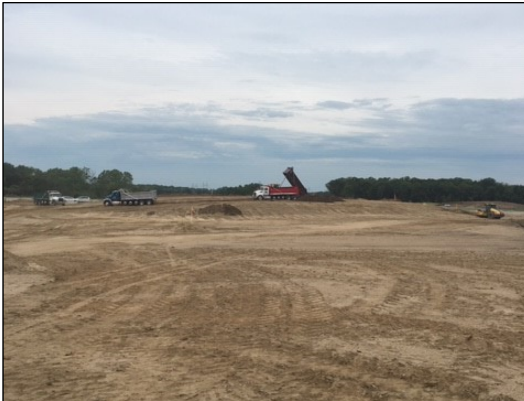
A look at the grading operation north of I-94. By the end of the July, crews had constructed approximately 10' of embankment
