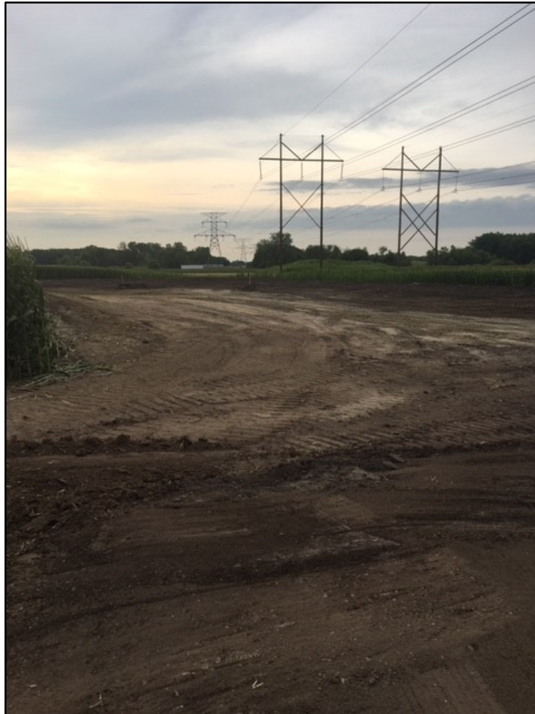
A look at the new pond on Brockton Lane just north of the Rush Creek Bridge. The area has been cleared and will be excavated
