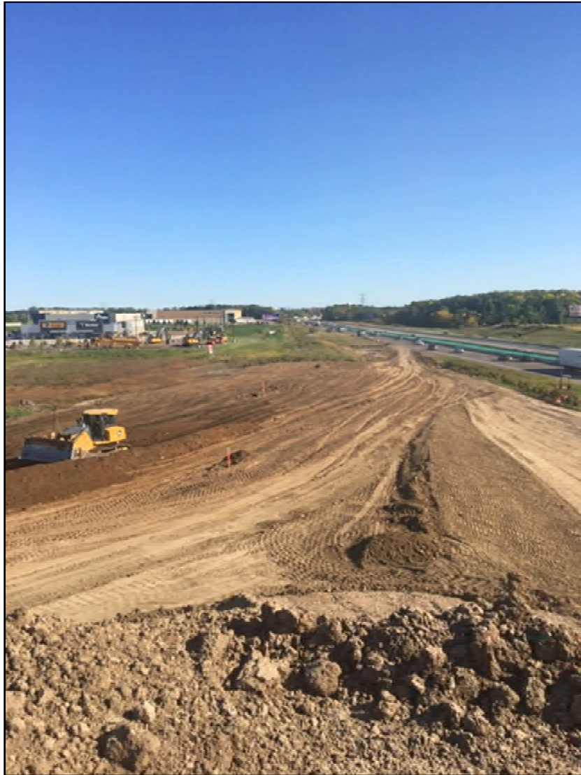
The grading operation north of I-94 looking east. This work is for the new WB exit ramp from I-94 to Dayton Parkway.
