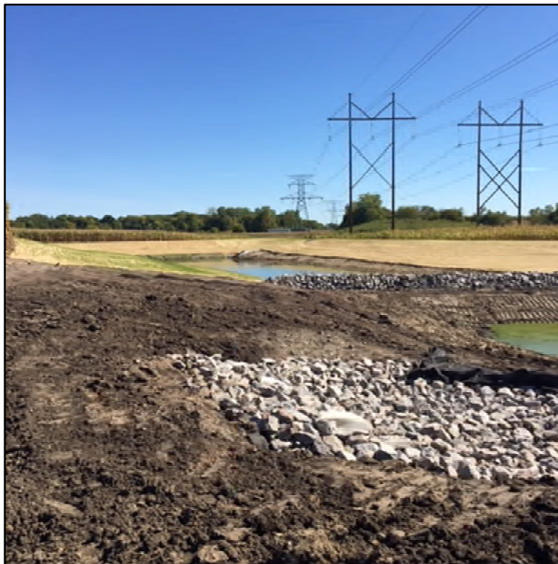
The new stormwater pond east of Brockton Lane just north of Rush Creek
