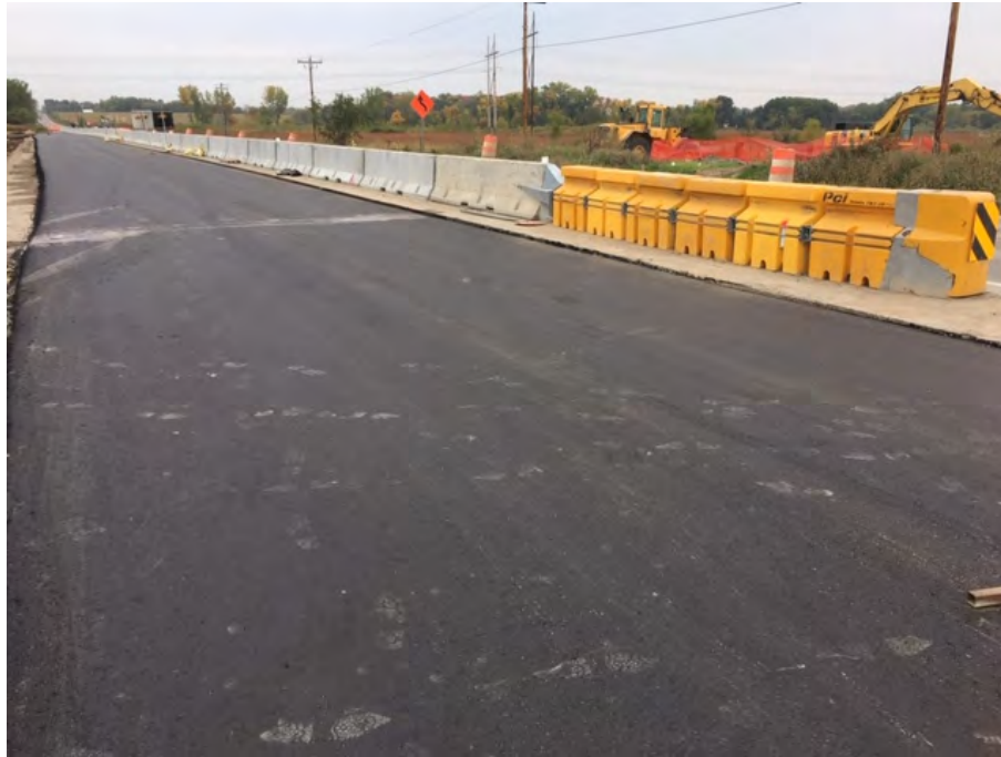
The new widened pavement on the northbound side of Brockton Lane looking south
