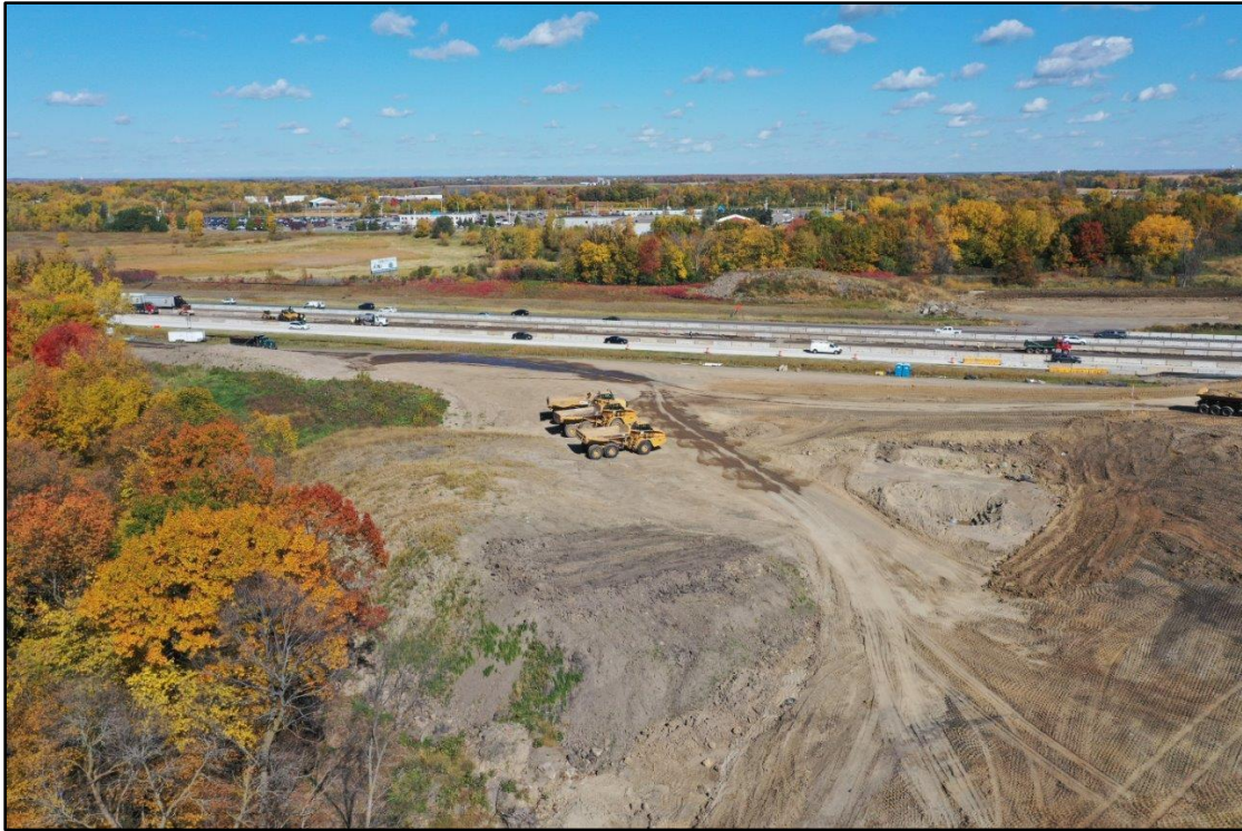
Drone photo of the Dayton Parkway embankment grading west of I-94 looking to the north.
