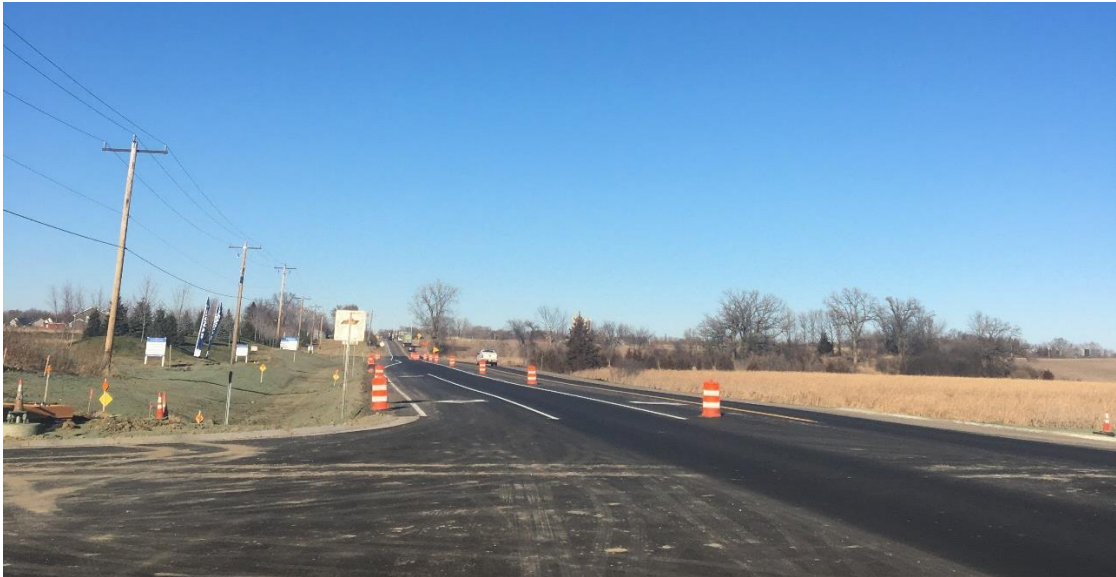
The completed widening of Brockton Lane looking North. The improvements include right and left turn lanes at the intersection of the new Dayton Parkway.
