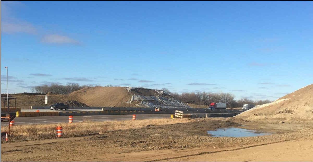
A view of the future Dayton Parkway bridge embankments on either side of I-94
