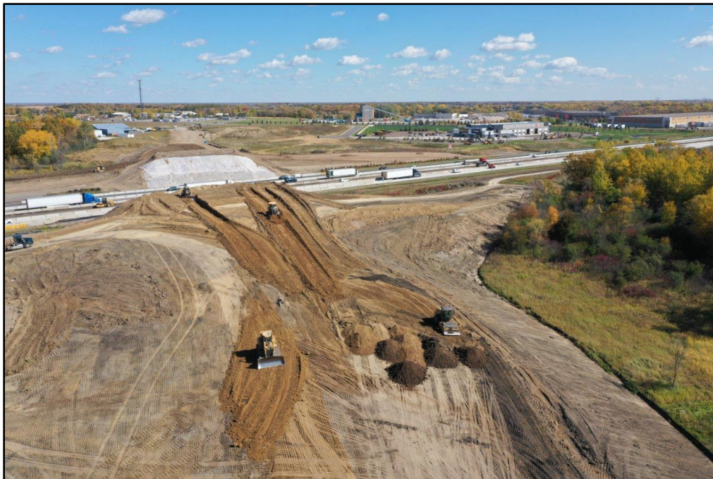
A view of the Dayton Parkway embankment grading west of I-94 looking to the east.
