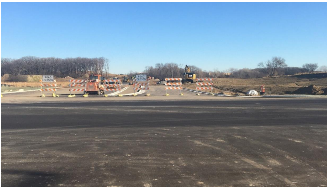
A view looking down the future Dayton Parkway from the Brockton Lane intersection.
