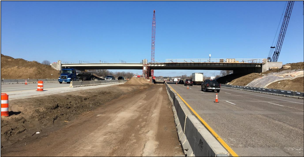
A view of the newly erected Dayton Parkway bridge beams spanning I-94 looking to the northwest.
