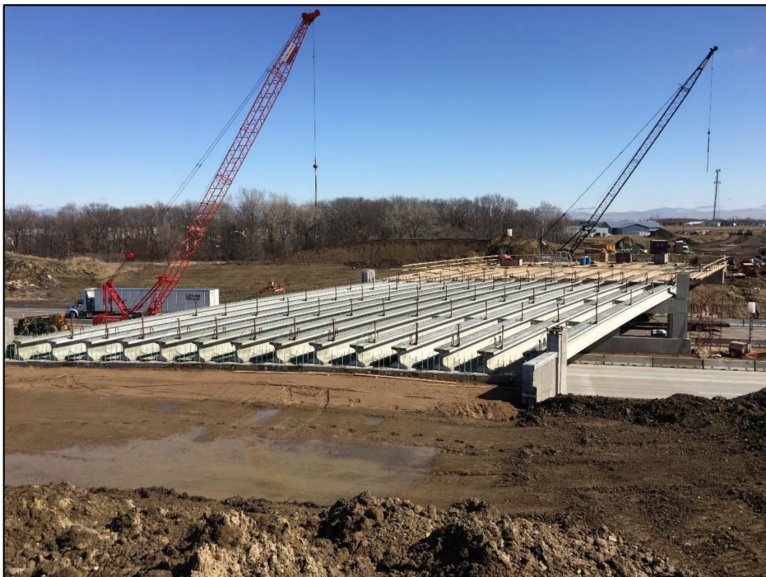
A view of the Dayton Parkway bridge beams over I-94 from the west abutment looking to the east.
