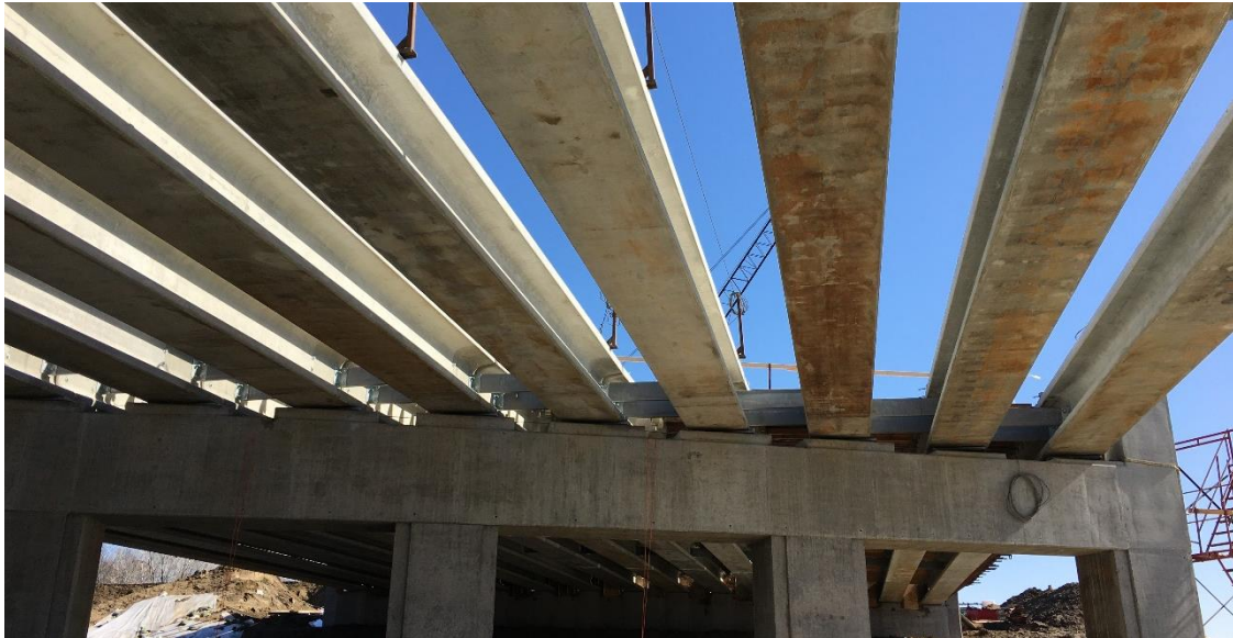
A view from I-94 below the newly erected Dayton Parkway bridge beams.
